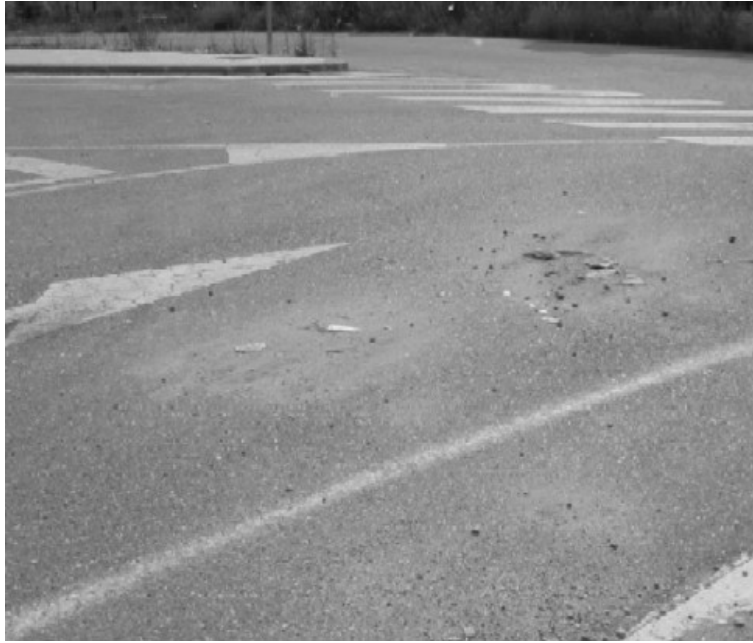
Figure 4: Dirt on road surface
