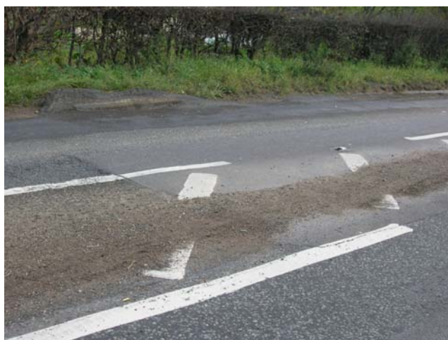
Figure 6 A350 Limber Lost, material movement due to tar contaminated pavement material
