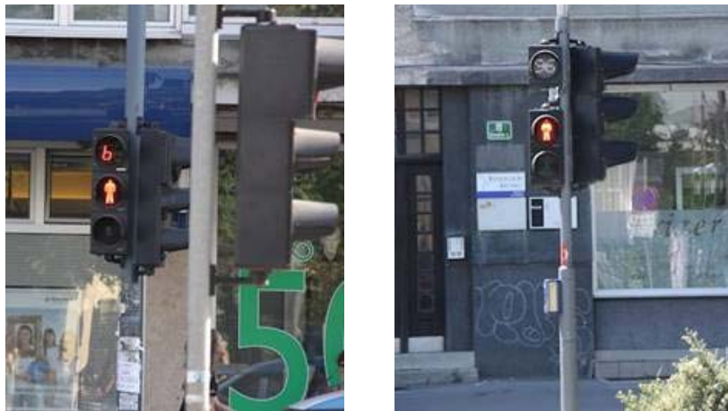
Figure 8 – Pedestrian traffic light equipped with countdown
